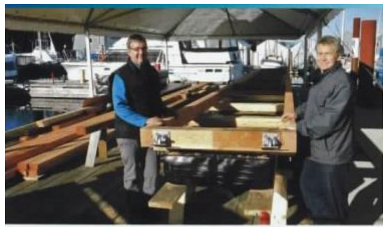
Marc Pettigrew and Brian Tilley working on a part of the 300 feet of new docks being installed at LMS in preparation for the busy summer season.
